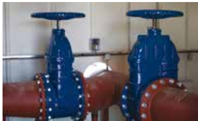
Pumps and Valves
